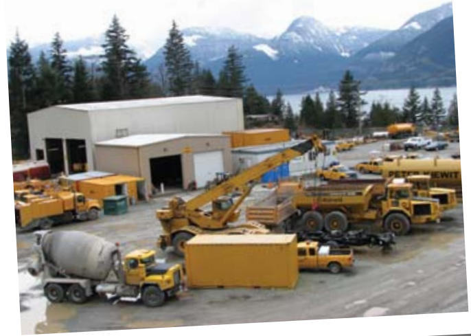
There are over 370 pieces of heavy equipment at work on the Sea-to-Sky Highway Improvement Project. This includes everything from pickups and cars to heavy-lift cranes, bulldozers and excavators and tracked rockdrills.
