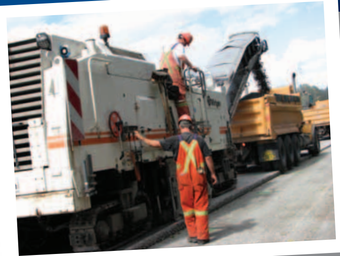
This powerful track-mounted cold milling machine can shave a 79" swath of old pavement and can be controlled to go as deep as 13". The machine is easily moved from location to location.
