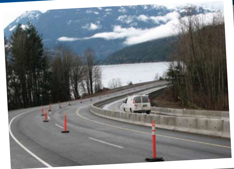
Photo shows temporary lane closure for line painting. New median barrier adds to the safety of this unique 1.9 kilometre three-lane hill and curve combination.
