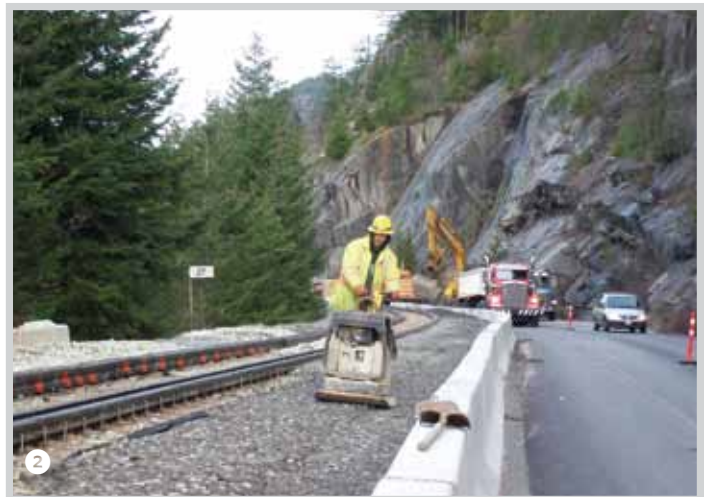
2 Asphalt contamination of the permanent rail ballast was prevented by placing filter cloth under the temporary road base, compacted in layers by various machines
