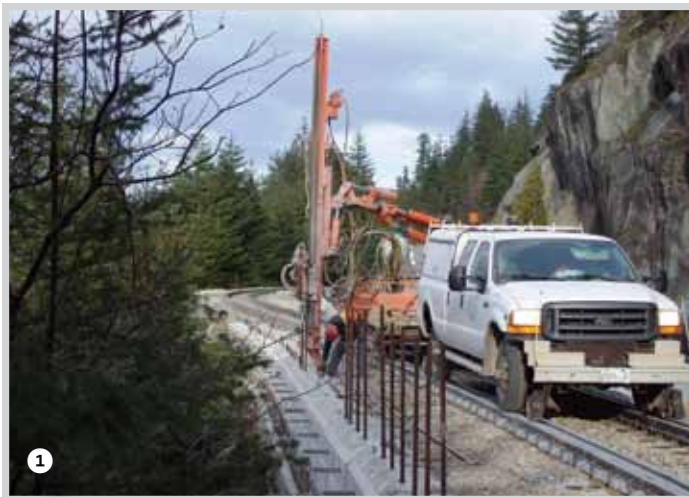
1 Where the rail bed had to be widened over steep areas, the ocean side of the road base is held in place by concrete lock block walls stabilized by steel rods.
