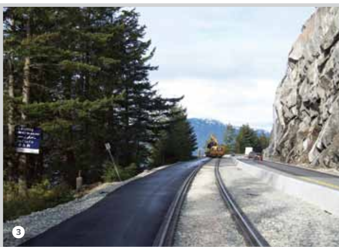
3 A drainage system underneath the track lane was installed to prevent water draining from it into the two highway lanes, and then concrete barrier was placed to retain fill and road base materials, and also to keep this lane separate as it enters and leaves the track.
