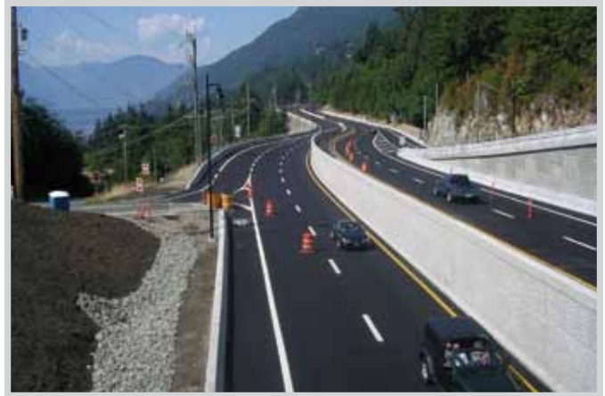
AFTER: View of Lions Bay from Kelvin Grove post-construction. The design is a split grade, multi-laned highway with 1.5-metre shoulders. Open Grade Friction Course (OGFC) or “quiet pavement” is laid throughout the community.
