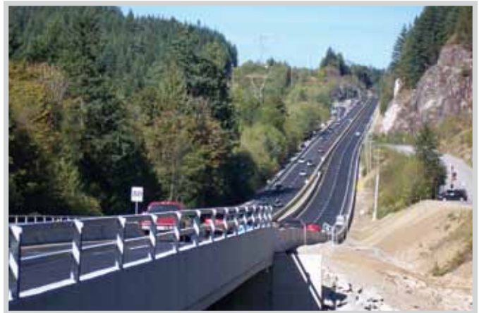
AFTER: Furry Creek hill post-construction as a four-lane highway divided by median barriers. Furry Creek Bridge and Middle Creek Bridge were widened to accommodate the doubling of capacity, centre line barriers and 1.5-metre shoulders.
