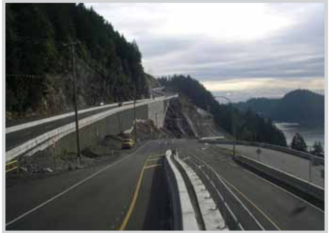
AFTER: Realignment of old highway at Pasco Road. View of new alignment on the left to Eagleridge Interchange. View of old highway to the right carries local traffic to Horseshoe Bay and BC Ferries. Improvements are part of a 4.6 km section of four-lane divided highway from Eagleridge Drive to North Junction.
